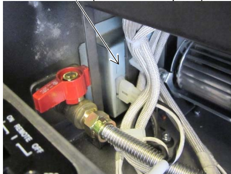
Junction Box (from inside fireplace)
